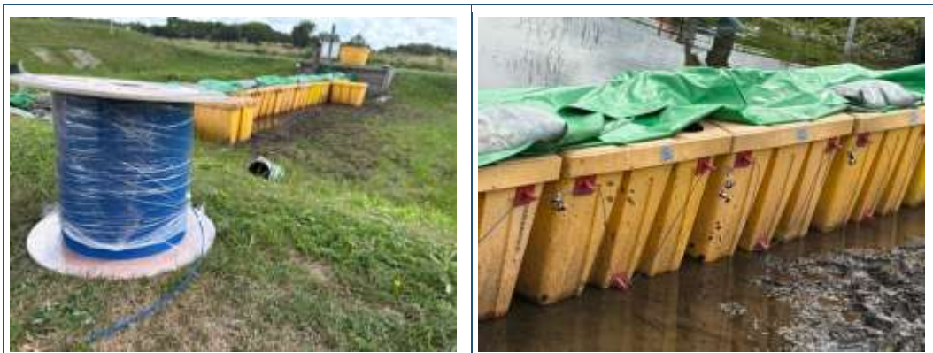
Figure 24 Fibre cable, clamps and pre-strain weights in between box cable connections.
