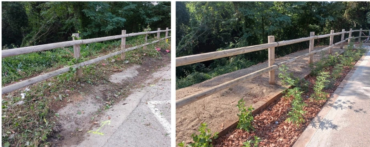
Figure 30. Left. Ditch before the bioswale that flooded giving problems to the adjacent parking lot. Right. New bioswale with direct infiltration capacity. Source: NATURALEA
