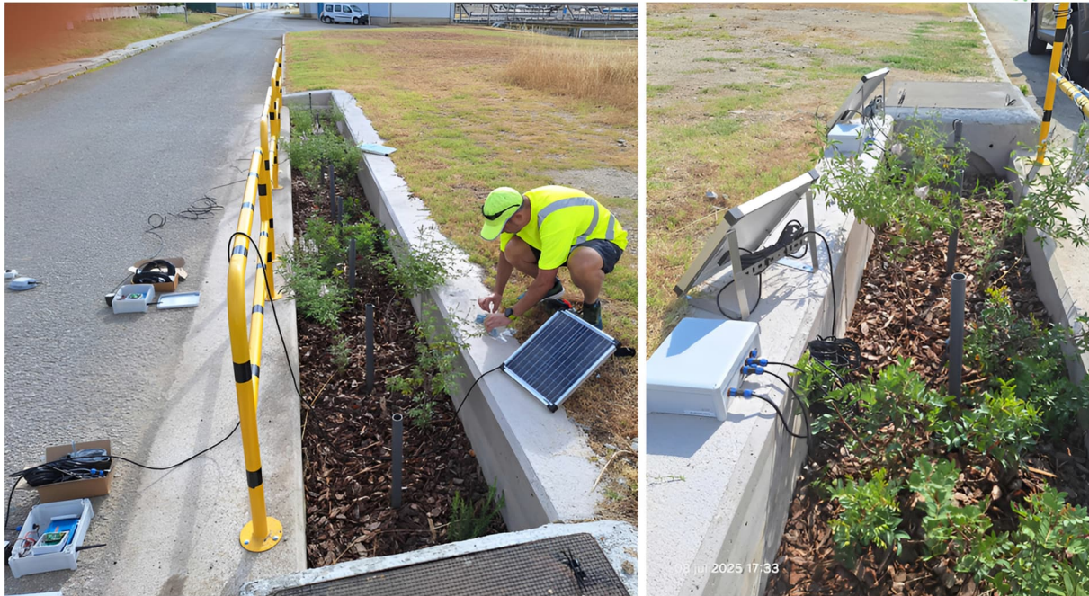
Figure 28. Detail of the centralizing boxes, before covering them (left) and after installation (right), for the sensors installed inside the bioswale unit in the URL. Source: NATURALEA
