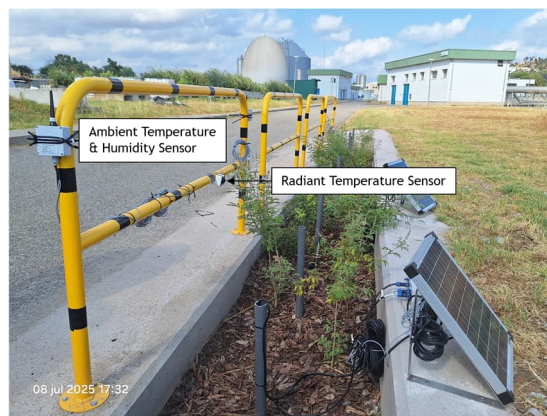
Figure 23. Sensors installed in a bioswale prototype at the URL. Source: MULTICLIMACT
