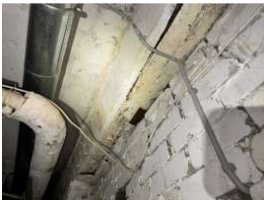
e) Corroded steel beam causing delamination of the protective concrete layer
