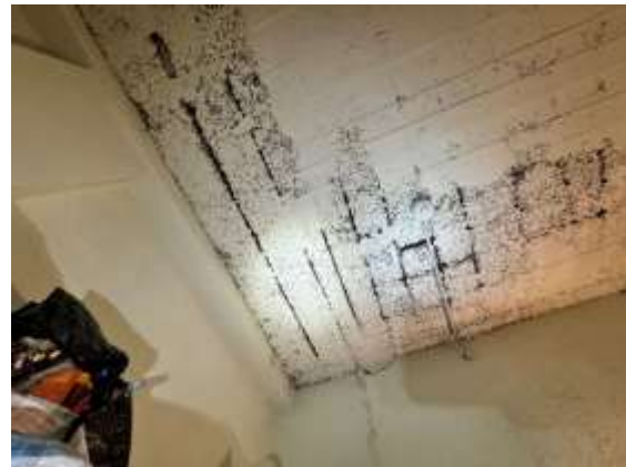
f) Exposed reinforcement due to poor concrete compaction during construction
