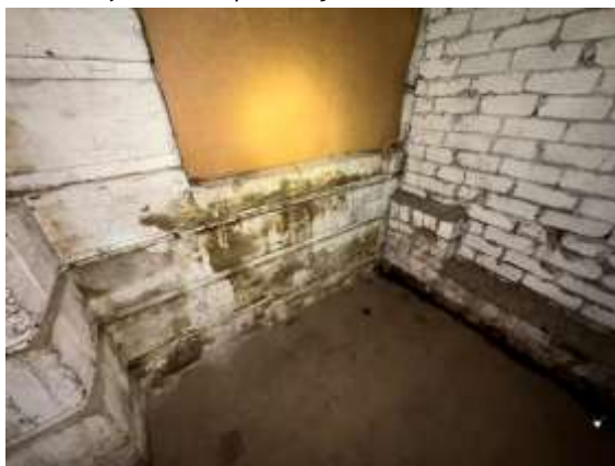
e) Moisture penetration into the basement through the old lightwells.
