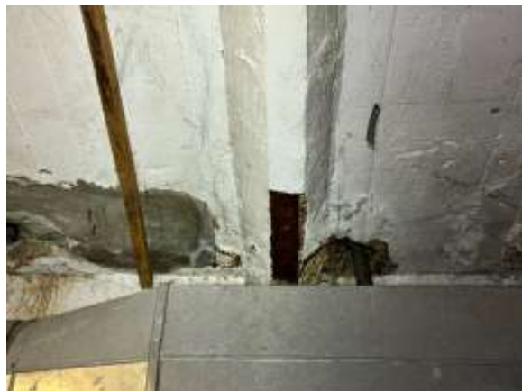
d) Corroded steel beam causing delamination of the protective concrete layer
