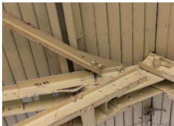
f) Upper truss elements near the roof ridge exhibiting localized deformations
