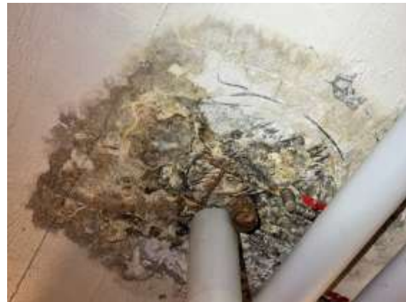
b) Moisture damage in the basement slab with corroded reinforcement
