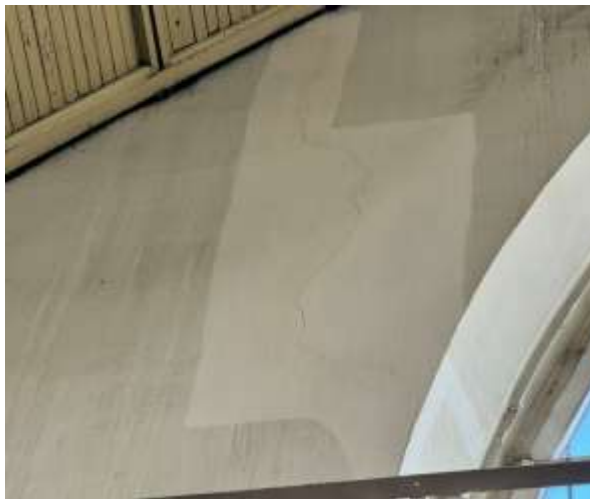
c) Cracks in the arched lintel (on the inside) with renovated finish - north wall of the building
