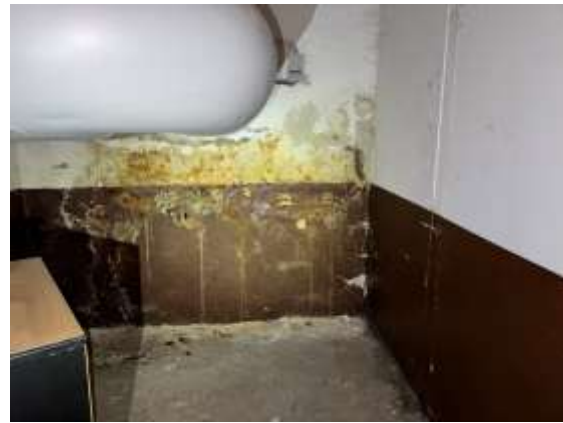
d) Damage due to prolonged moisture saturation in the basement walls of the building
