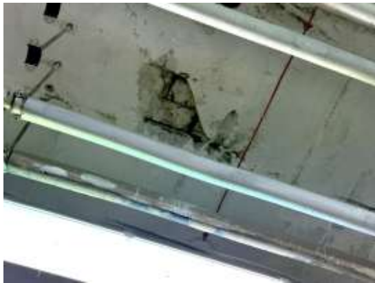
e) Locally corroded slab reinforcement with spalling of concrete
