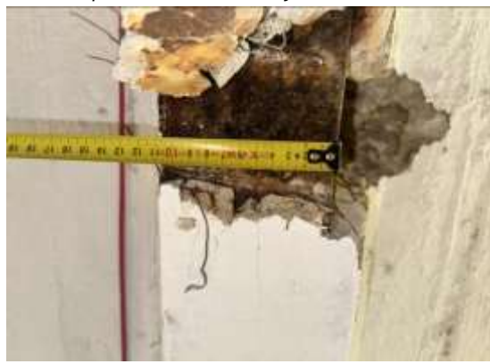
f) Superficial corrosion damage in the bottom flange of the steel beam
