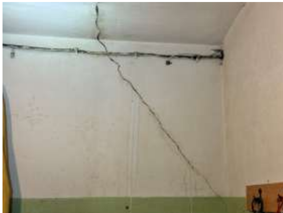
c) Diagonal cracks in the stairwell wall extending from the expansion joint in the slab
