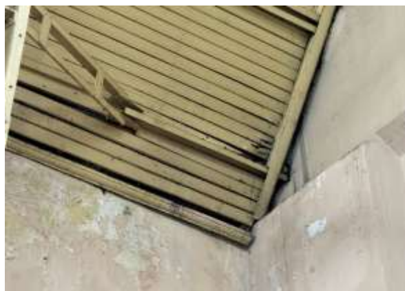
h) Wooden plank ceiling with signs of precipitation moisture infiltration
