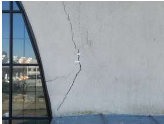
a) Cracks in the arched lintel - north side of the building
