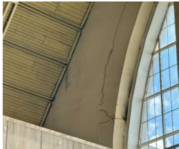
d) Cracks in the arched lintel (on the inside) - south wall of the building
