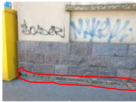
f) Damage in the plinth of the building potentially allowing moisture penetration into the basement
