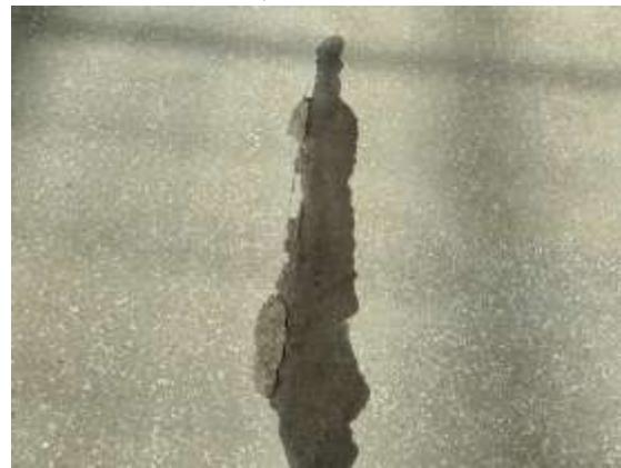
d) Floor cracks and surface layer chipping on the first floor
