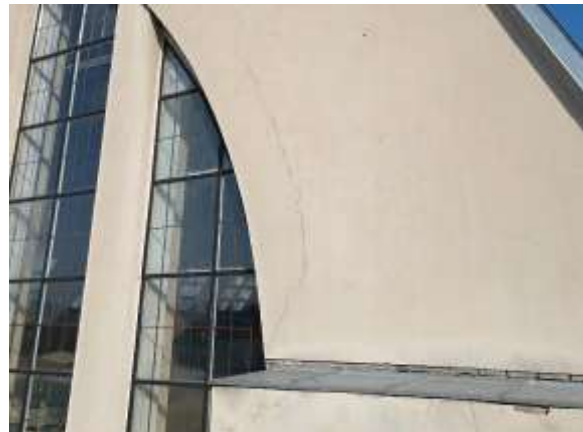
b) Cracks in the arched lintel - south side of the building.
