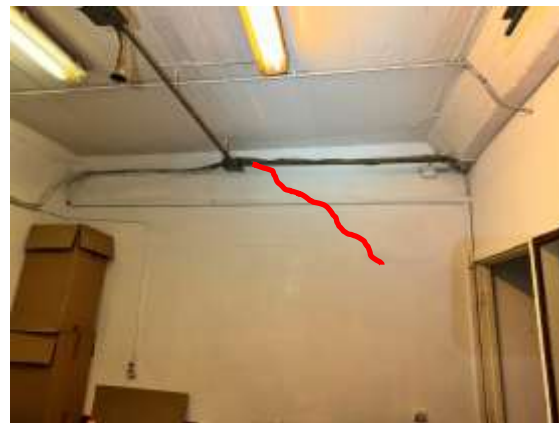
b) Diagonal cracks in basement walls
