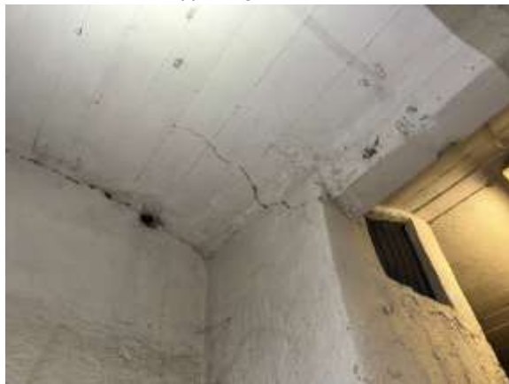
c) Cracking in the slab and foundation walls at the support of steel beams
